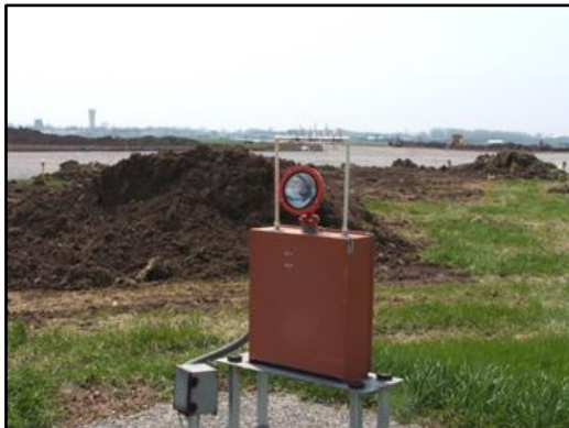
Runway 27 REIL stands ready to assist pilots in locating the runway.
